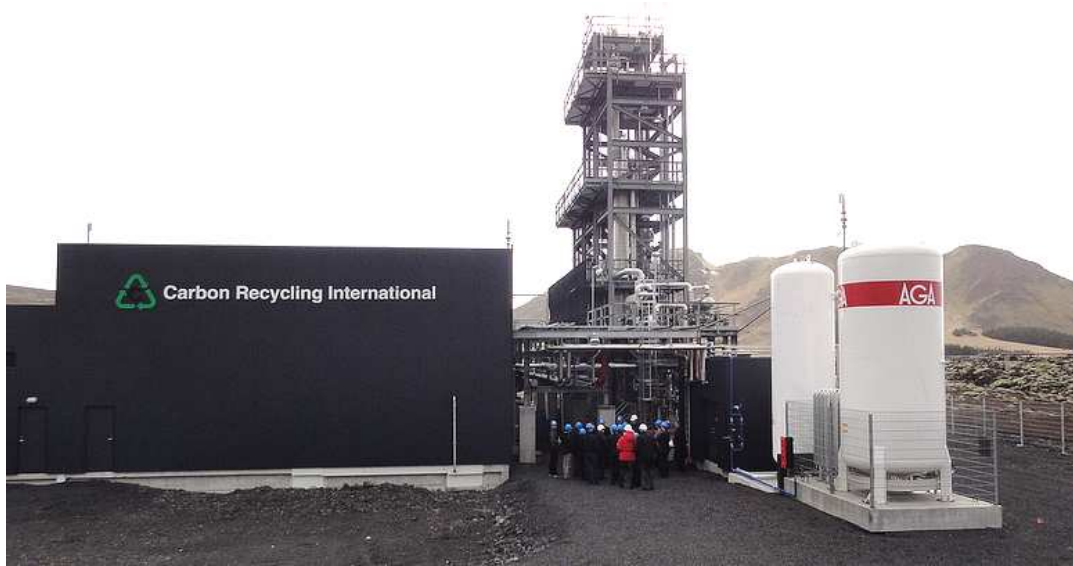
Abbildung 17 CO 2 -to-Methanol-Anlage, Svartsengi Geothermal Power Plant, Reykjanes, Island (Bild: Carbon Recycling International Opening 2012, © ThinkGeoEnergy, Lizenz CC BY 2.0)
